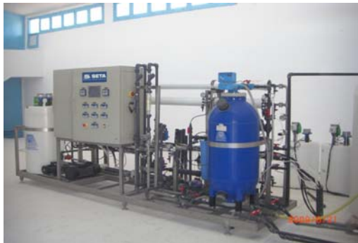
Figure 1: Reverse-Osmosis Desalination Plant
