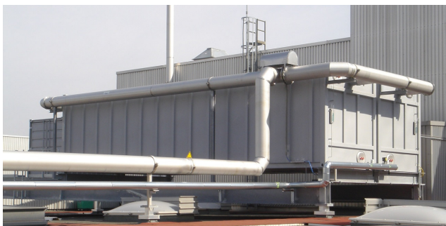
Figure 5 A real installation of a modern biofilter [REINLUFT]
