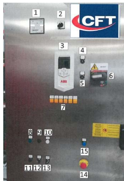
Figure 3: Machine electrical panel.
