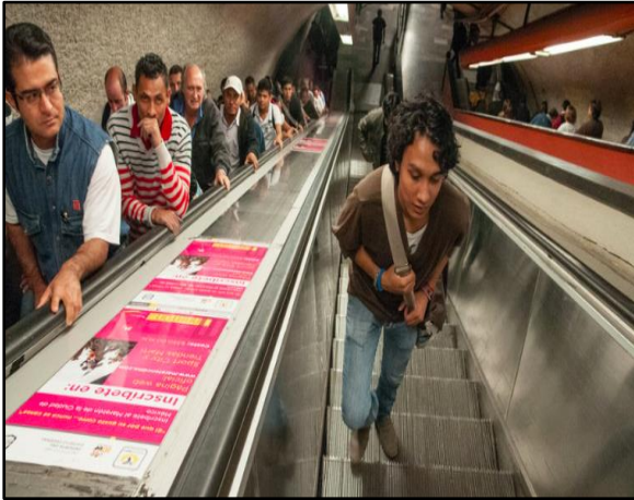
Figure 2: Passengers on escalators in TACUBAYA subway station when one escalator failures
